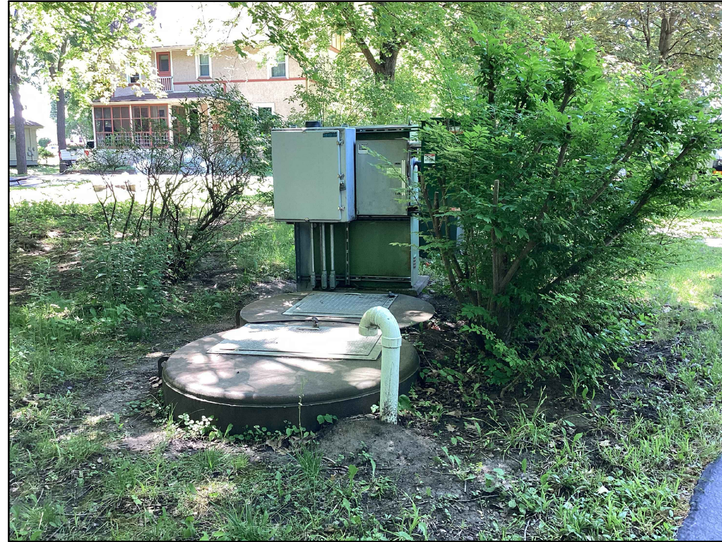
LIFT STATION AREA
