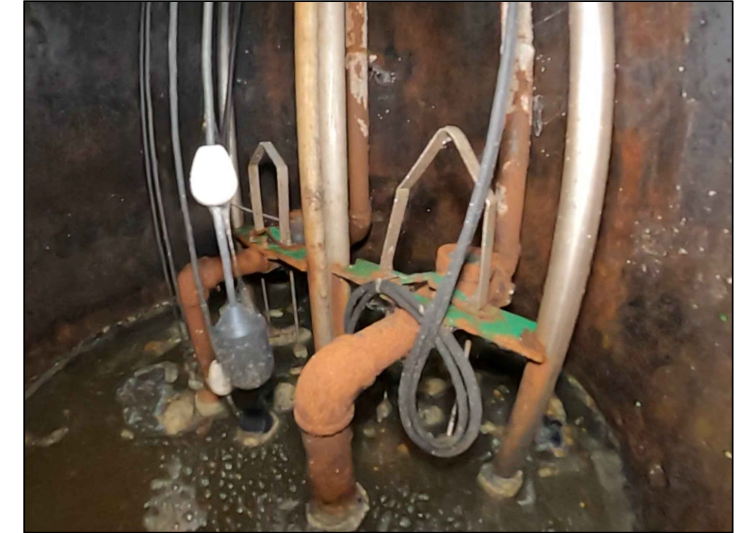
WET WELL DISCHARGE PIPE CORROSION
