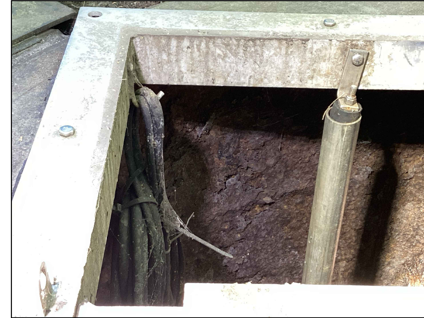
WET WELL WALL CORROSION
