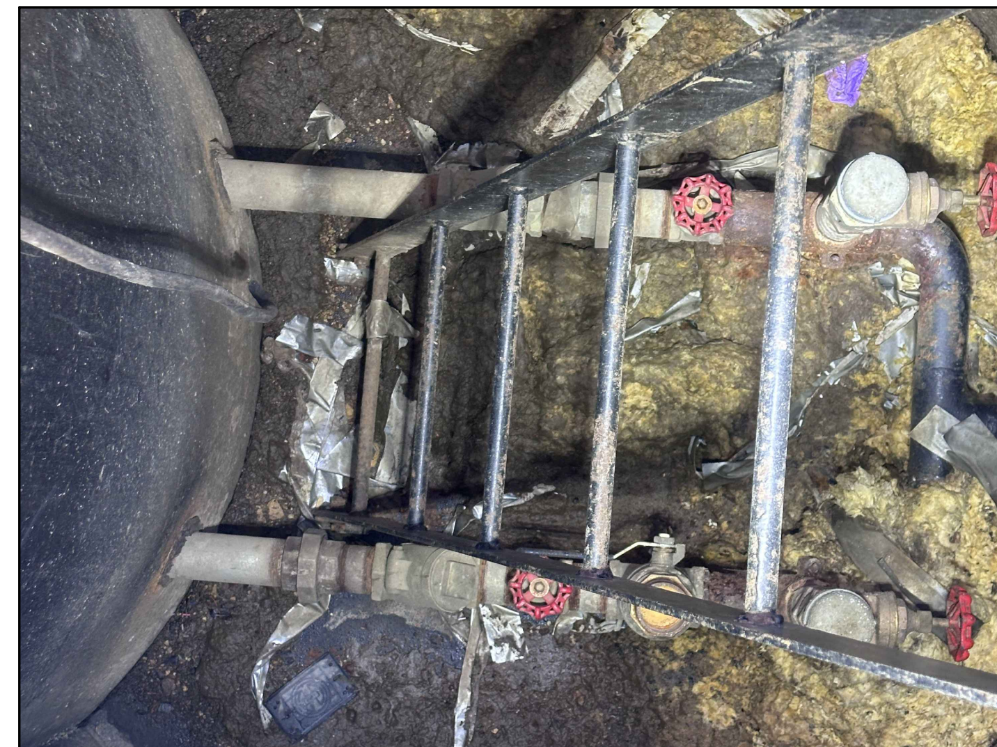
VALVE VAULT CLOSE-UP
