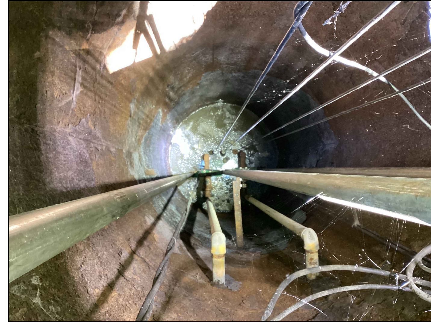
WET WELL TOPSIDE FACING NORTH
