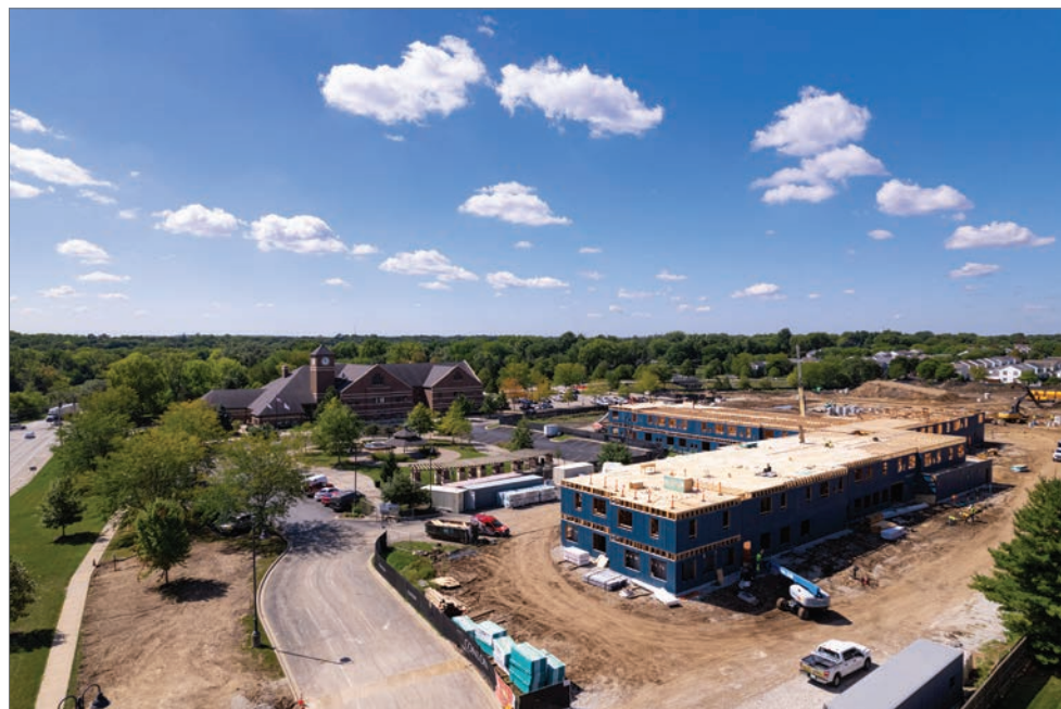
Just north of Village Hall, The Brant at Oswego development will provide seniors with options for independent living, assisted living and memory care. Completion is tentatively scheduled for summer 2024.
