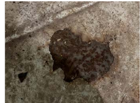
Corrosion of Condensate Platform
