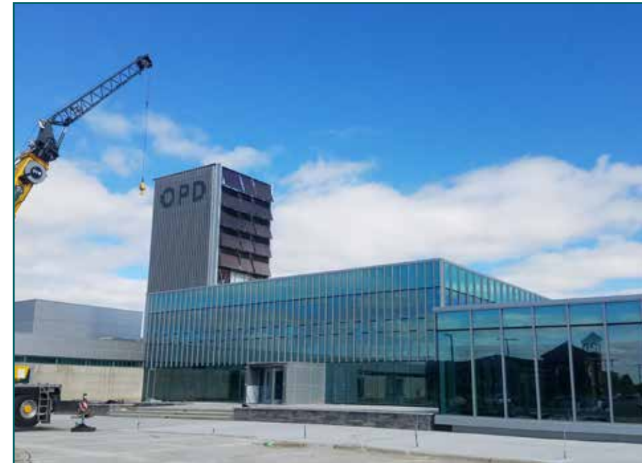
The new headquarters of the Oswego Police Department nears completion on Wooley Road. The new facility includes space for organizations like the Kendall Co. Health Department and Mutual Ground to provide critical support services for a healthier, safer community.
