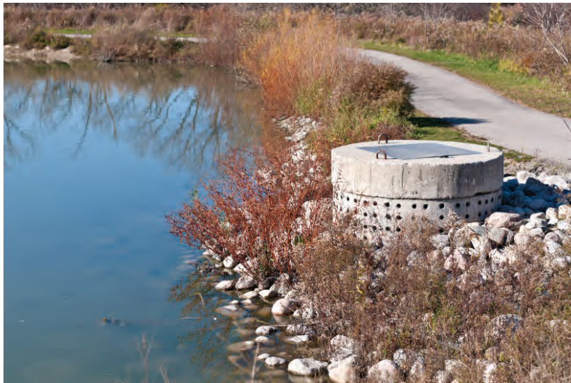
A perforated concrete pipe forms part of a stormwater management system in a suburban pond.
