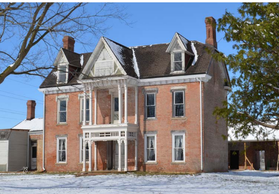
THE MARBOLD FARMSTEAD IN ITS HEYDAY (TOP), AT ITS MOST DETERIORATED (MIDDLE), AND NOW ON ITS WAY TO BEING FULLY RESTORED (BOTTOM, 2017). THANKS TO THE HISTORIC MARBOLD FARMSTEAD ASSOCIATION FOR THE TOP AND MIDDLE PHOTOS
