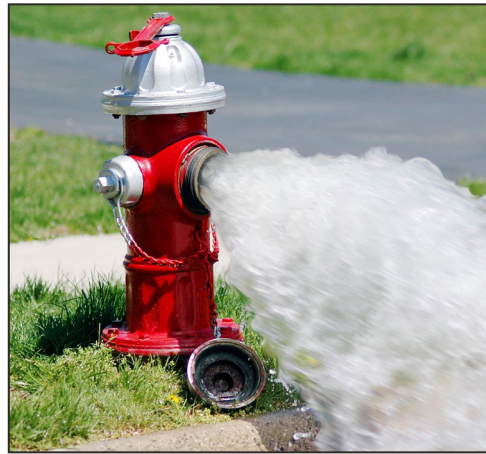
Water main flushing flushes iron deposits and helps pull fresh water all the way through the line.
