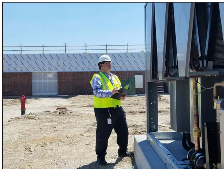
Facilities Manager Steve Raasch inspects recently delivered equipment at the new Oswego Police facility. His position is split between Yorkville and Oswego, saving both communities money.
