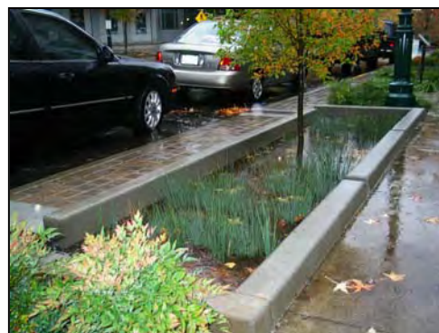
Typical parkway/ sidewalk with stormwater infiltration planters
