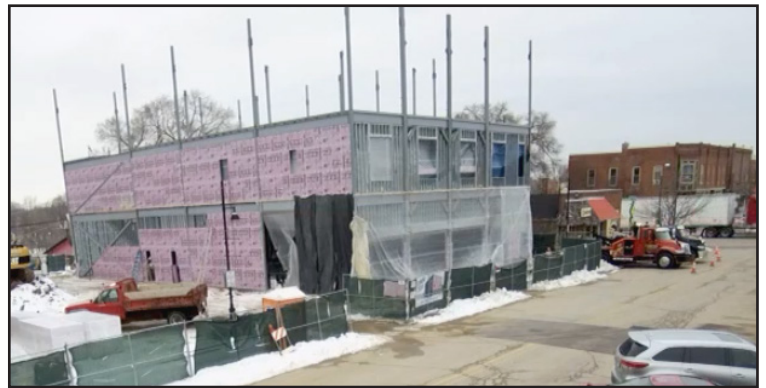
Construction has kept moving all winter long at 113 Main Street. You can watch progress on both this project and The Reserve at Hudson Crossing live-streamed on our downtown construction page, GoOswego.org/coming-soon .
